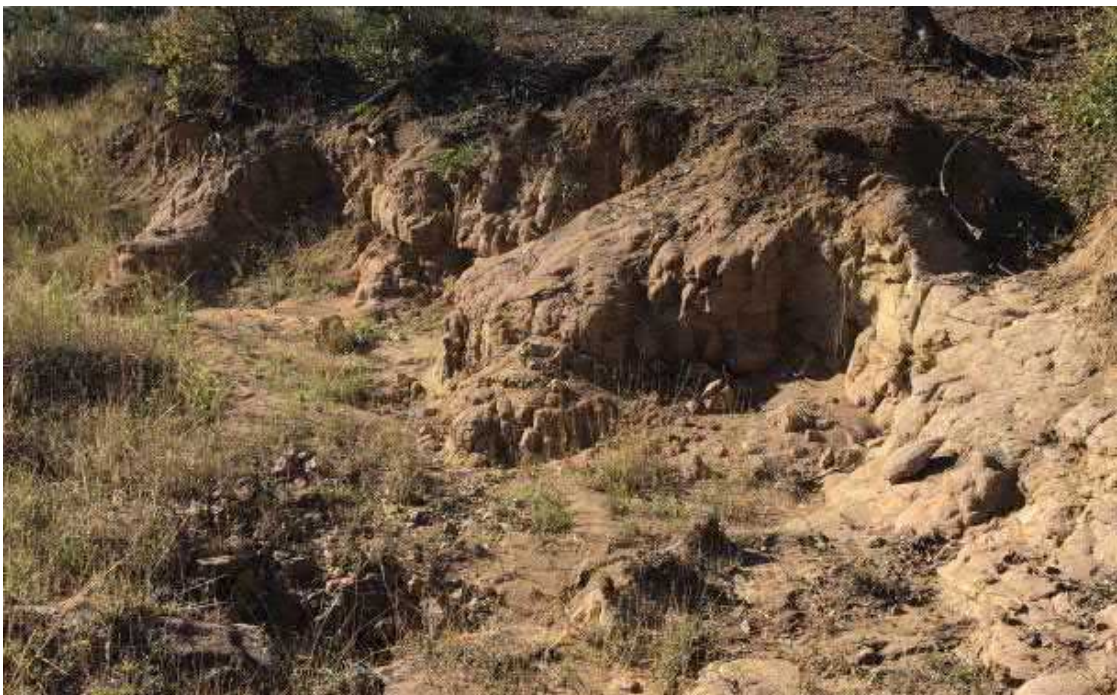
Photo 2-2 Erosion on tributary of Horse Creek
