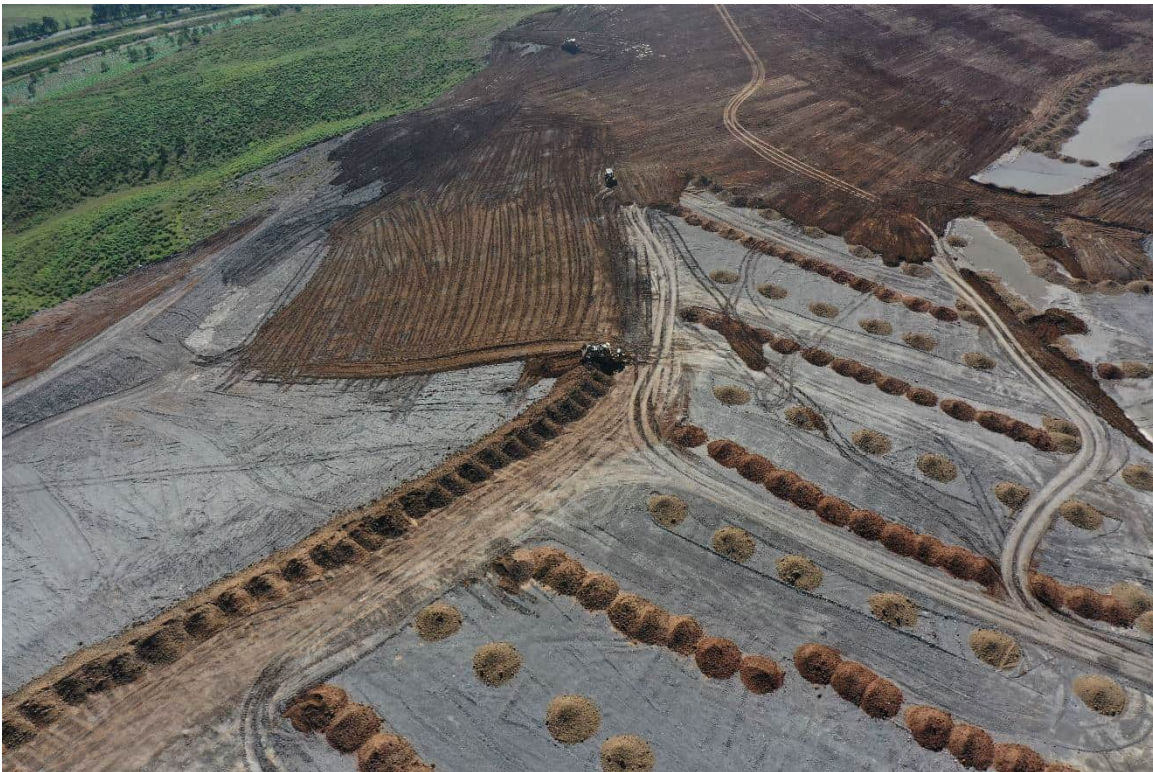
Figure 8 Bulk shaping and topsoil spreading at VD4 and VD5 Box Gum Woodland rehabilitation
