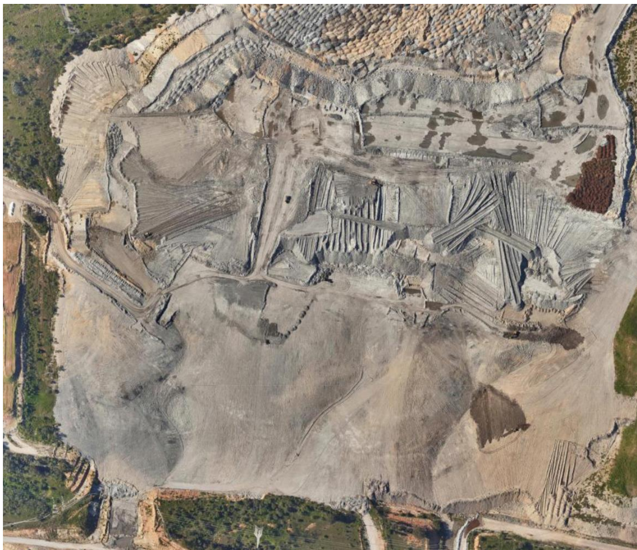
Figure 1 Rehabilitation works underway at Saddlers North at the southern end of the mine.
